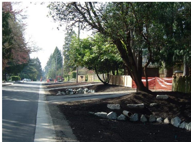
Streetscape in Seattle in construction showing swale/infiltration areas and sidewalk on other side of street, photo provided by Tetra Tech
